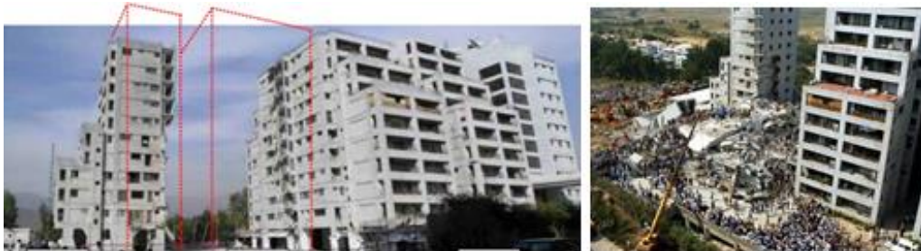
Fig. 2. Margalla tower collapse in the 8th October 2005 earthquake (Shoukat et al. , 2015a)
